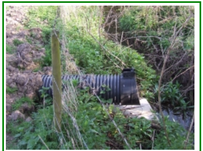
Outfall - 150mm pipe with flap valve
