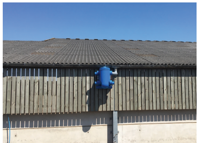
Southfields Rainwater Harvesting
